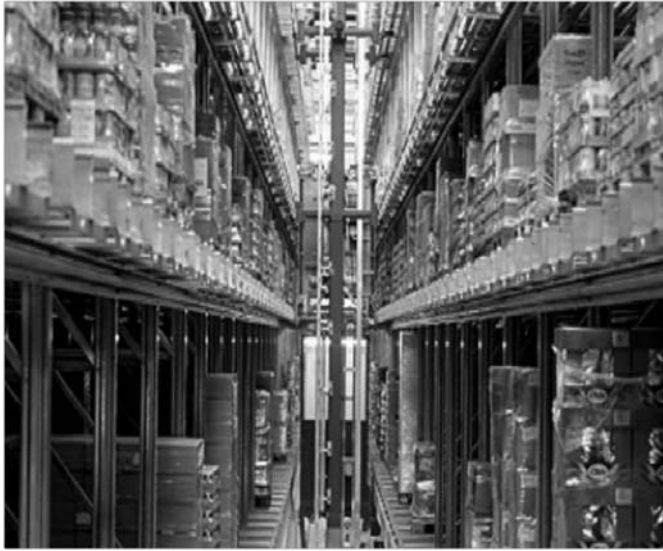
Figure 5.8 Automated Storage and Retrieval System
